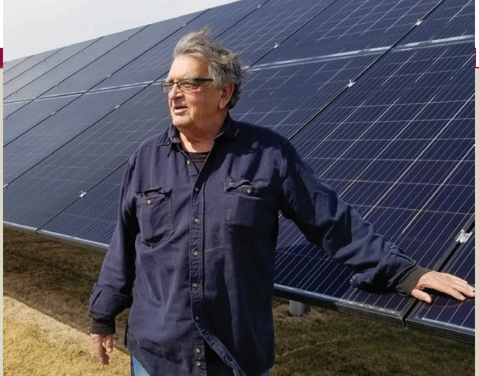
In his acreage north of town Doug Pitlik stands with his 38-panel solar array. "I produce and use a lot of electricity," Pitlik noted. In his acreage north of town Doug Pitlik stands with his 38-panel solar array.
