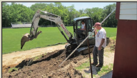
Nick Boren '02 and Mike O'Brien (general contractor) begin the process of digging new footings.
