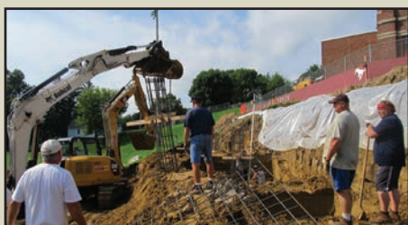
Mike O'Brien, Kevin Whitman '76, Wayne Hormann '85 and Aaron Hormann '86 wait for Nick Boren '02 to set one of 21 rebar columns to be assembled with the rebar grid in the footing.
