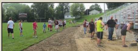
Future alums and community members lay sod and carry bricks for a retaining wall under the bleachers on one of the volunteer days.
