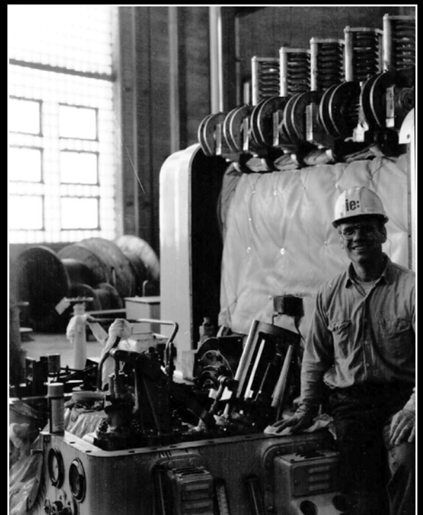
1995 - Chris Stoltz ('63) works inside the Sixth St. Power station in Cedar Rapids
